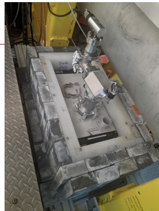
Rad shielding of DS1 roughing pump
